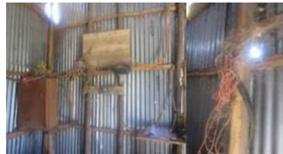
Fig2.Current poor electric cable installation practice in pumping stations.(Source: on site visit)
