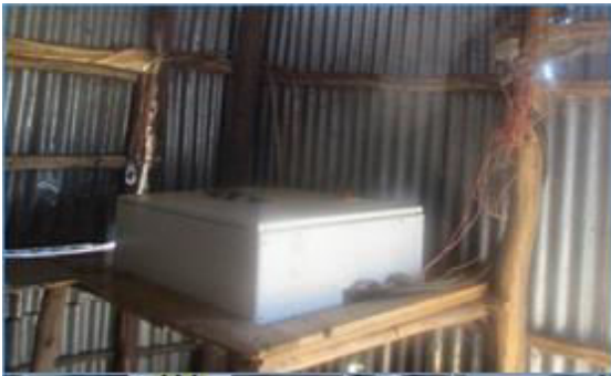
Fig. 4. Current installation practice of pumping station control box. (Source: on site visit)
