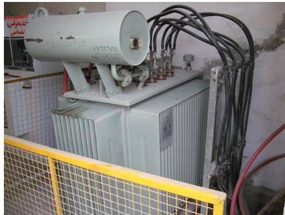
Figure 4. The picture of 400 kVA distribution transformer
