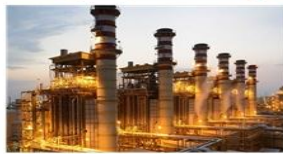
Combustion and Power Generation(2)
